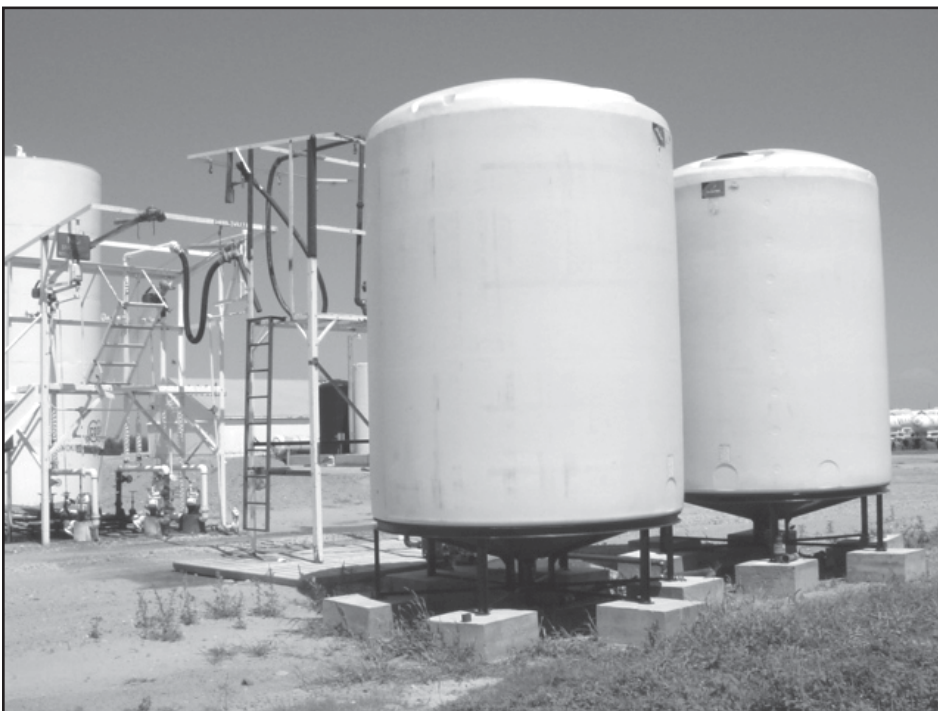
B100 Biodiesel Plant
